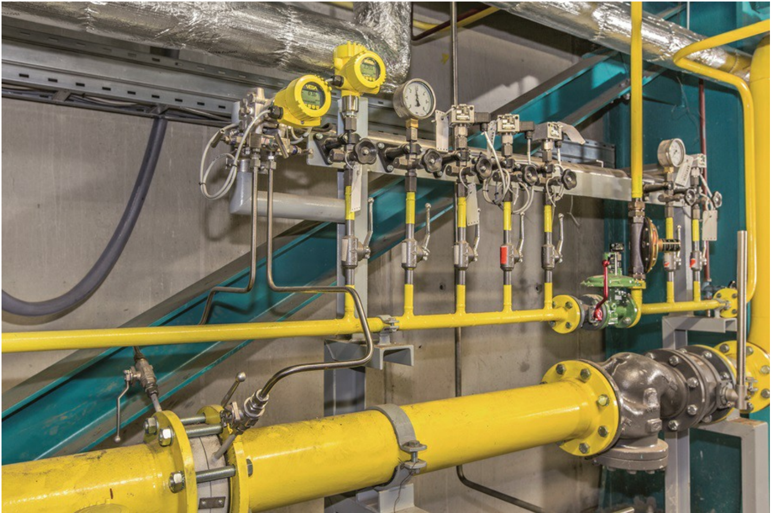
Flow measurement via an orifice plate and mechanical differential pressure. The static pressure is measured by an additional sensor.
