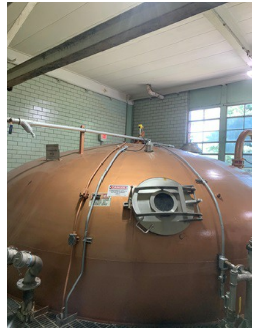
A bright yellow VEGAPULS 64 radar sensor perched atop this massive copper fermenter vessel measures level to output volume.
