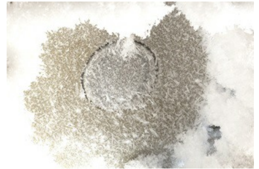
A thick layer of frost built up on the radar antenna (center circle) and on the flange.
