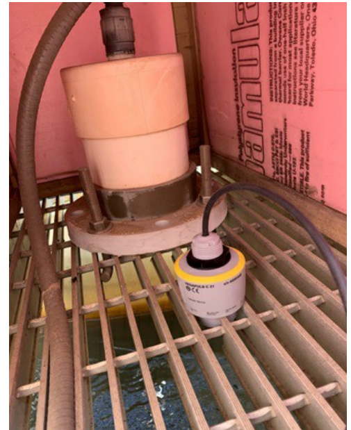
A radar level sensor and an ultrasonic transmitter are installed side-by-side to compare their performances.
