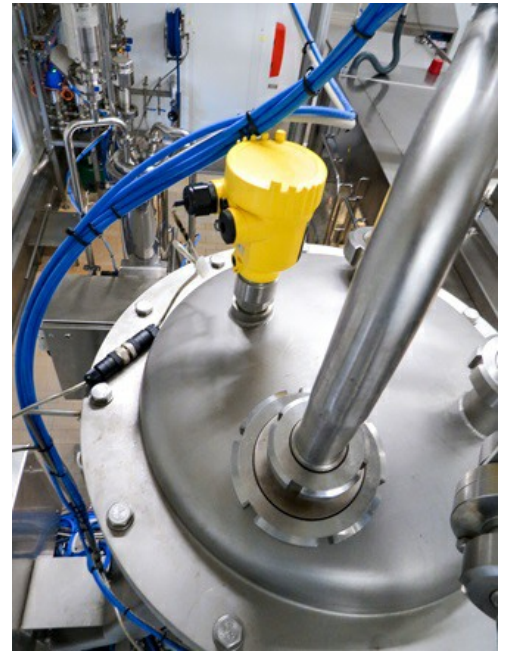
VEGA sensors control the level to keep the yoghurt filling process running smoothly.
