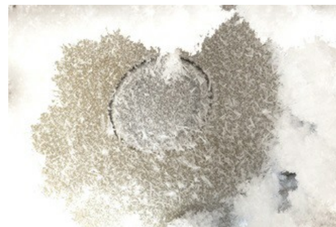
A thick layer of frost built up on the radar antenna (center circle) and on the flange.
