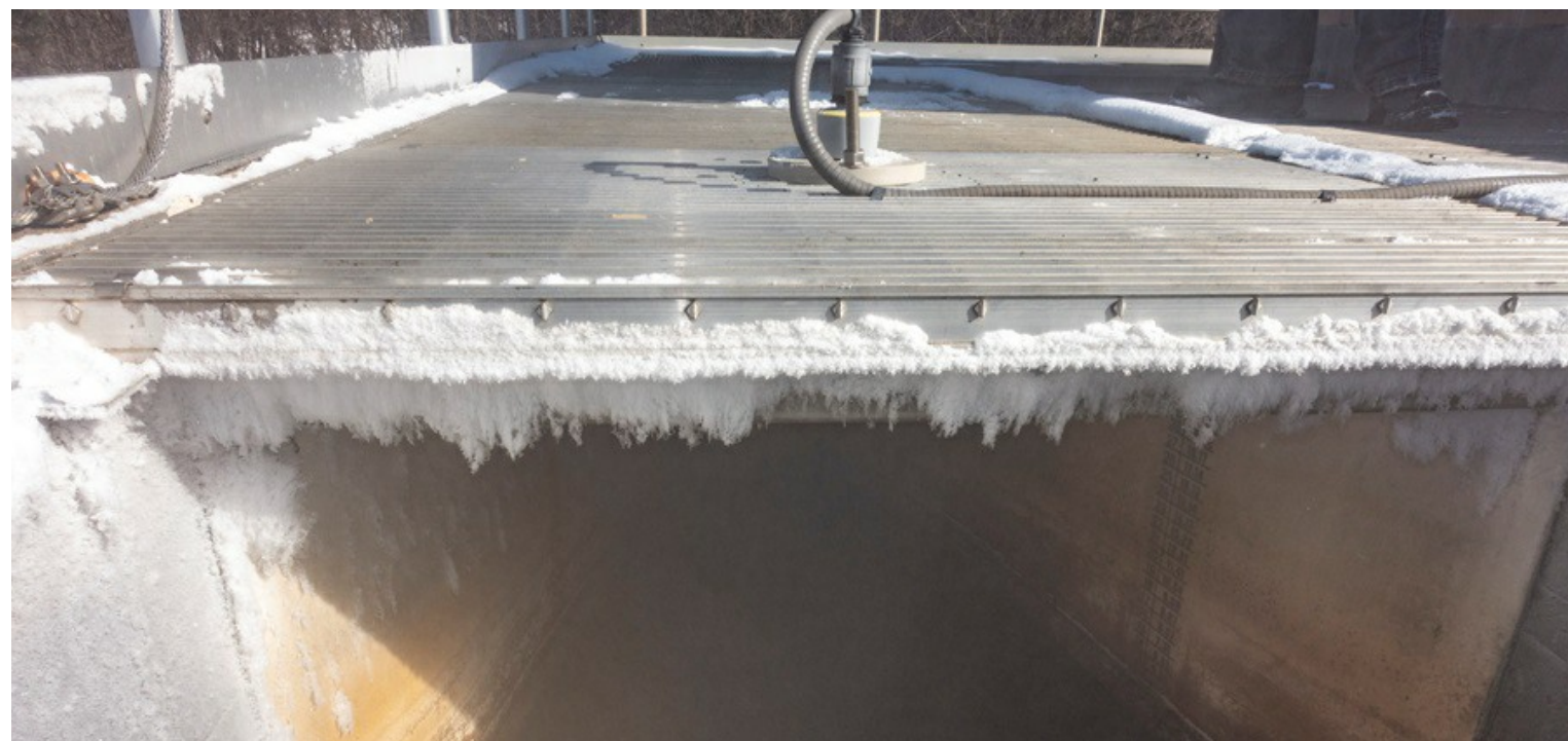
The influent channel gets frosty during the cold winter months, making it a challenge for some level measurement instrumentation to make a reliable, accurate measurement in the flume.
