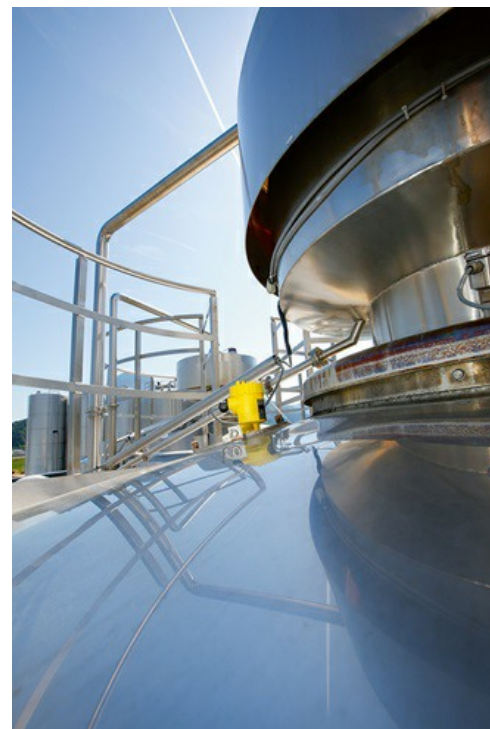
VEGAPULS 64 measures the level reliably in the whey tanks.
