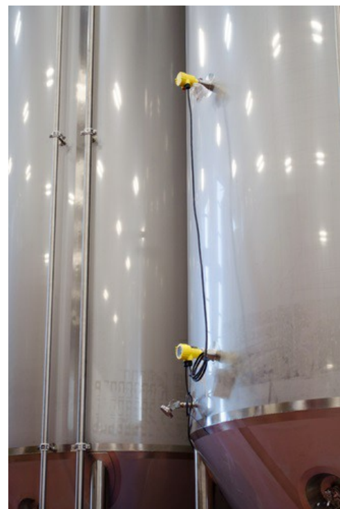
Two VEGABAR pressure transmitters connected by a cable are installed on the vessel – one near the bottom and another near the top.
