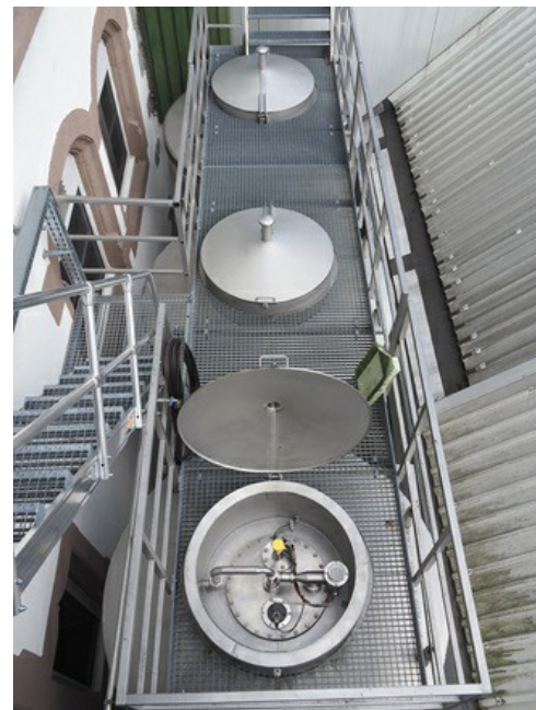
View of a VEGAPULS 63 radar level transmitter on one of the maturation vessels.
