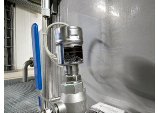
Measuring point with VEGABAR 82 and "Second Line of Defense".
