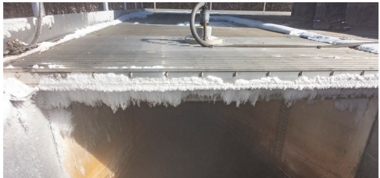
The influent channel gets frosty during the cold winter months, making it a challenge for some level measurement instrumentation to make a reliable, accurate measurement in the flume.
