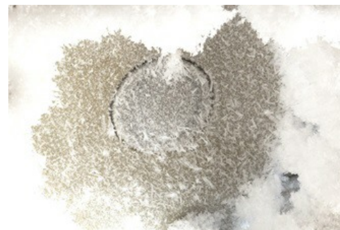
A thick layer of frost built up on the radar antenna (center circle) and on the flange.
