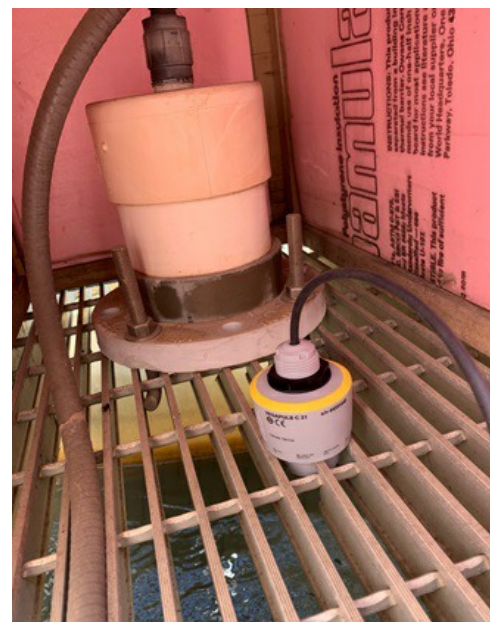
A radar level sensor and an ultrasonic transmitter are installed side-by-side to compare their performances.
