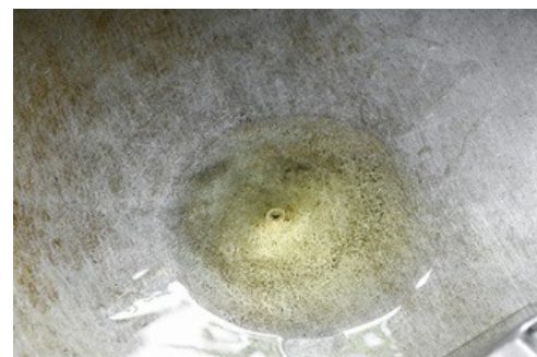
Oil on the tank floor. At low levels, it is very difficult to measure oils or other liquids accurately.
