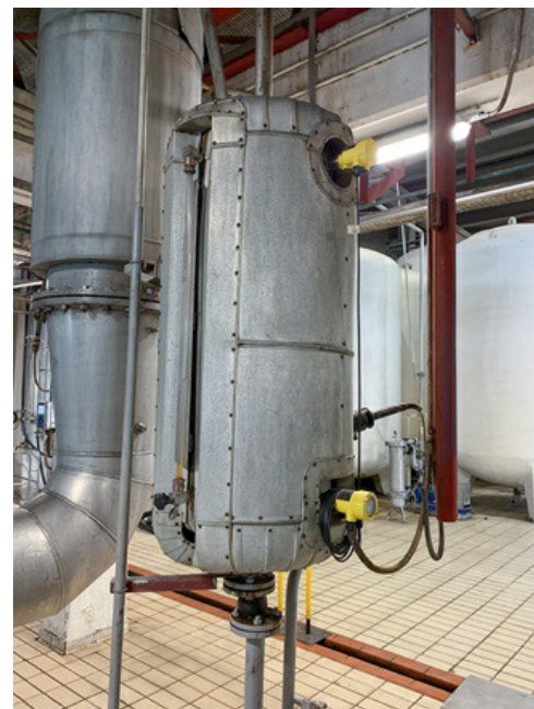
Pressure sensors of type VEGABAR 82 monitor the concentration of tartaric acid, an important component of grappa.
