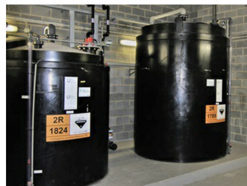
Chemical tanks for storing acids and alkalis.
