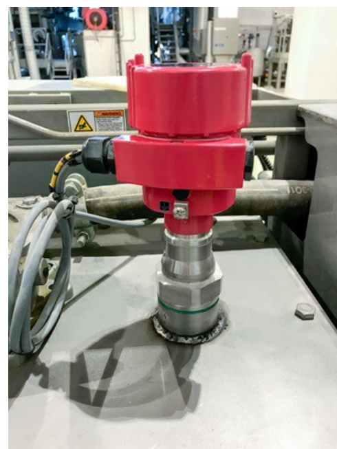
Notice that these VEGA sensors are not yellow, but the typical Progroup red.
