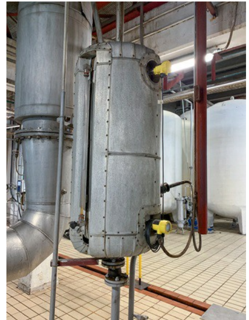
Pressure sensors of type VEGABAR 82 monitor the concentration of tartaric acid, an important component of grappa.
