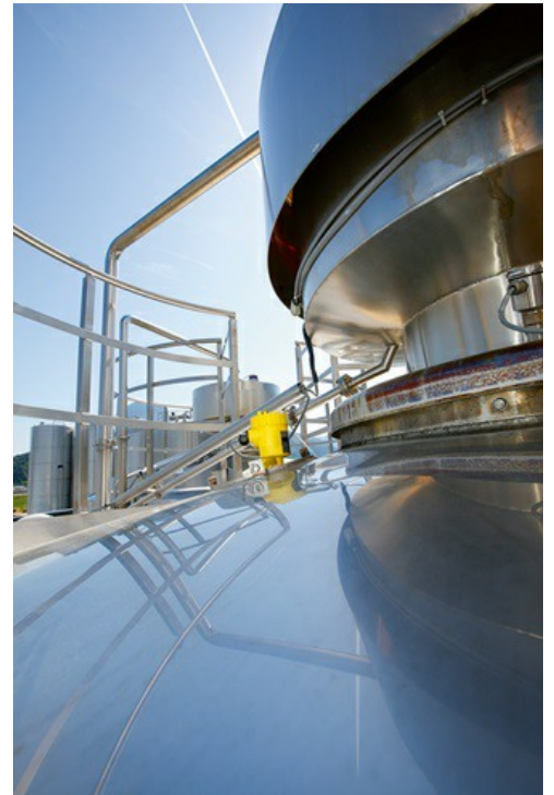
VEGAPULS 64 measures the level reliably in the whey tanks.
